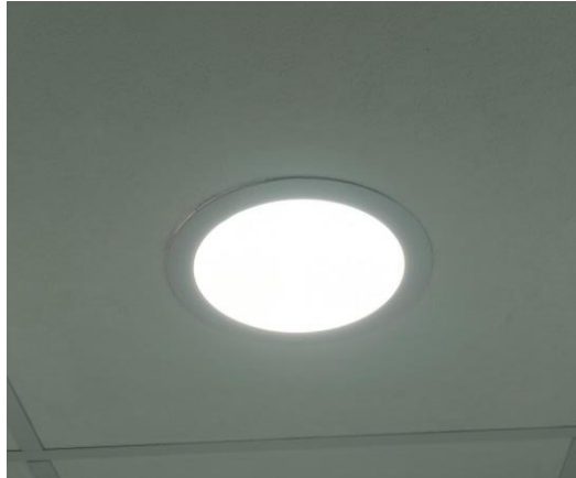
Fig. 28 Foco Downlight LED
