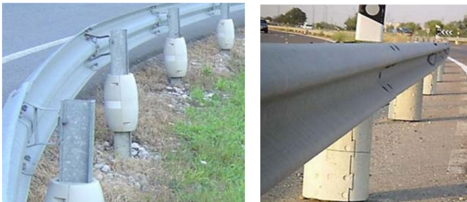
Figure 2. Examples of discontinuous motorcyclist protection system installed on European roads [7].
