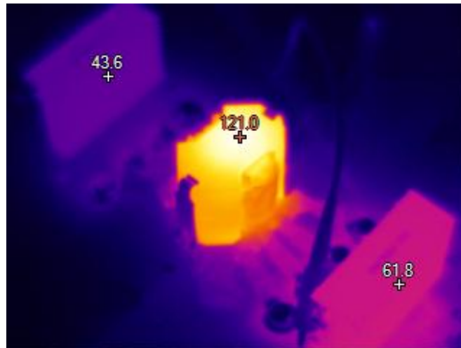
Figure 41. Thermal image of DCX 3 main hotspots. From left to right: Rectifier diode heatsinks (D 1 ,D 2 ), Transformer, MOSFETs (M 1 ,M 2 ). Temperature in °C.
