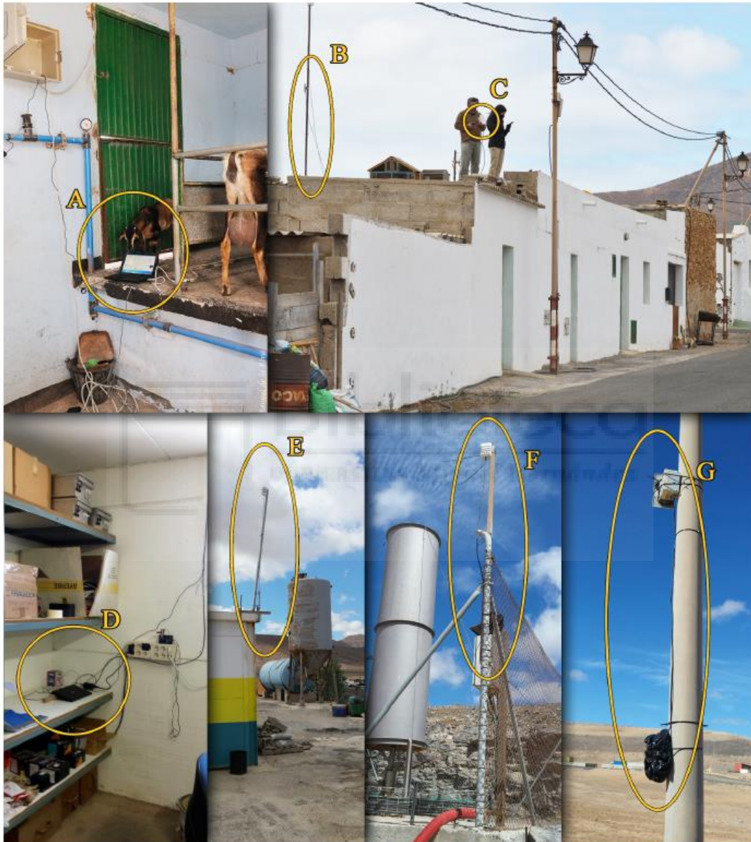
Figure 7. Details of the required system for the proper functioning of UvABiTS devices. (A) Laptop installed close to the main supplementary feeding station serving as base station number 1. (B) Antenna connected to laptop 1. (C) Relay used during the installation of a supporting relay for the base station 1. (D) Laptop installed close to the garbage dump serving as base station number 2. (E) Antenna connected to laptop 2. (F) Relay installed inside the garbage dump supporting base station 2. (G) Another relay installed inside the garbage dump supporting the base station 2. Photography © M. de la Riva (top) and L. Gangoso (bottom).
