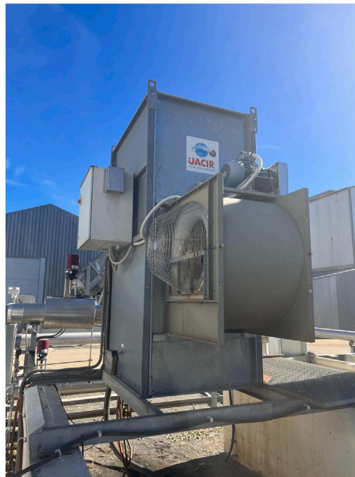
(b) Back view of the WCT
