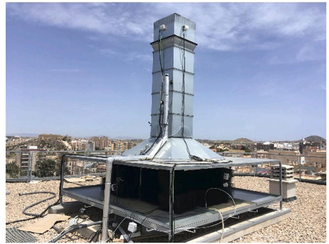
Fig. 1. Built prototype of the inverted cooling tower.
