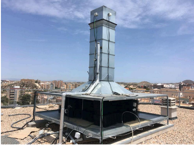
Fig. 2. Built prototype of the inverted cooling tower.
