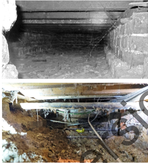
Figure 2: Images of typical underfloor environments where the registration is difficult due to their characteristics.
